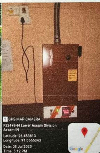
Incinerator for Sanitary Pad Disposal
